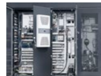
Climatized electric cabinet with easy access.
